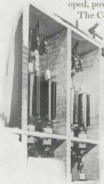
Low tension, 13,200 volt switches
