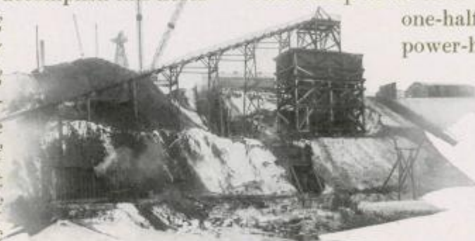
Complete Concrete Mixing Plant at Work
