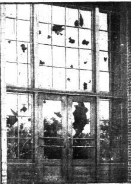
Main entrance to Kohler office, showing damage to glass.
